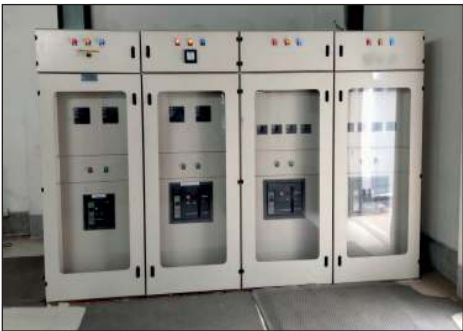
Main Distribution Board (MDB) Danish Foods Ltd.
