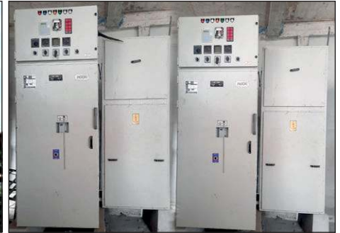
33KV 1250A & 800A Indoor Switchgear Famous Steel & Re-rolling Mills Ltd.
