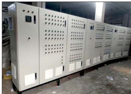
Low Voltage MCC Panel Noman Group at Mulaid, Gazipur
