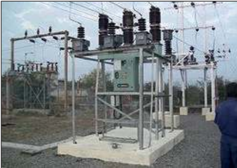
33KV 1250A Outdoor type VCB Safui Alam Steel Mills Ltd.
