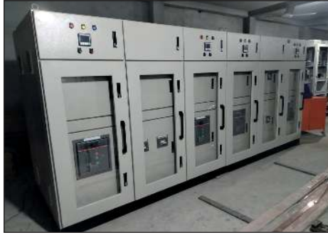
Main Distribution Board (MDB) Metrocem Ispat Ltd.
