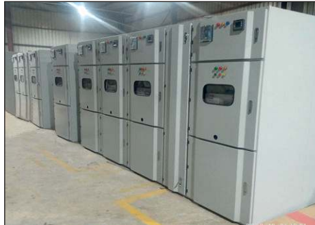
11KV 1250/630A HT Switchgear Panel Narayanganj Wasa
