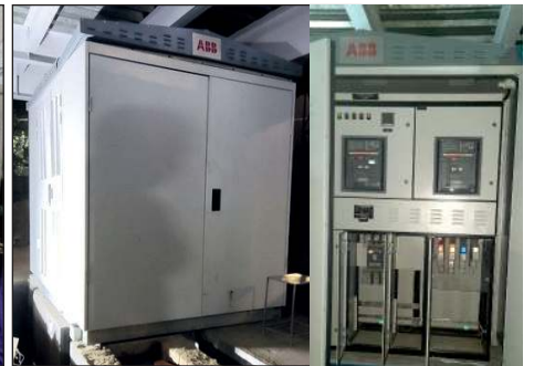
11/0.415KV 800KVA ABB Compact Sub-Station Elegant Square at Gulshan Avenue
