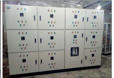
Motor Control Center (MCC) FKL Spinning Ltd.
