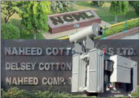
11/0.415KV 2500KVA Transformer with OLTC Delsey Cotton Spinning mills Ltd.
