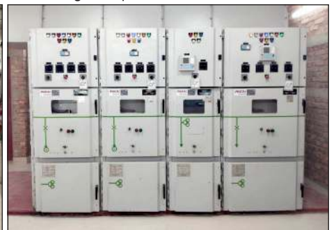
11KV, 1250/630A, HT Switchgear Panel (VCB) Based & Sons Steel Re-rolling Mills At Kodomtoli
