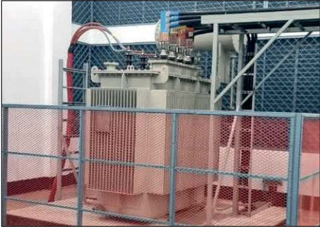
11/0.415 KV 1250 KVA Sub-Station Medicon Pharmaceuticals Ltd.
