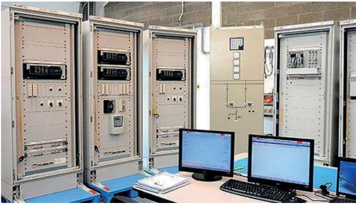
Industrial Substation Automation
