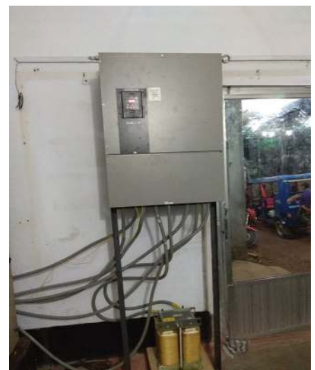
CNG Station 260kW Hitachi Inverter
