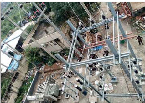
33/11/0.415, 5000KVA Sub-Station Echoknits Ltd. at Kaliakair
