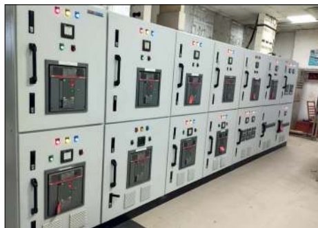
13500A Low Voltage Switchgear Echotex Ltd. at Polli Biddut, Chandura, Gazipur.
