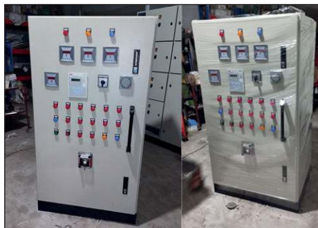
Relay Control Panel SAS Steel Mill
