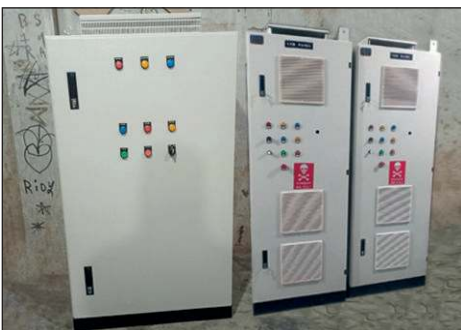
Saidaabad Water Treatment Plant 450KW VFD Panel
