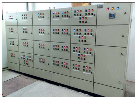
Low Voltage MCC Panel Far East Group
