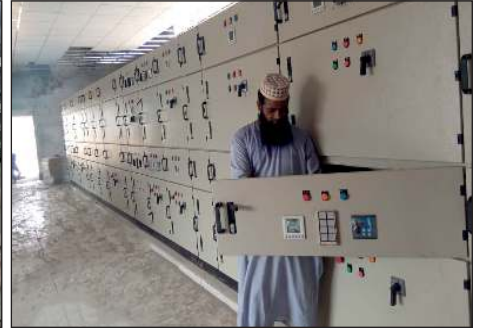
Low Voltage Switchgear with Bus-coupler Pretty Composite Textiles Industries Ltd.
